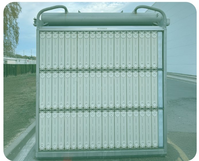
Image 2. Reused UF membranes from the Sant Joan Despí DWTP.
