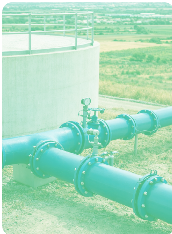
Reclaimed water distribution system (stock image)
